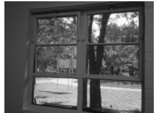
Windows Painted Shut
